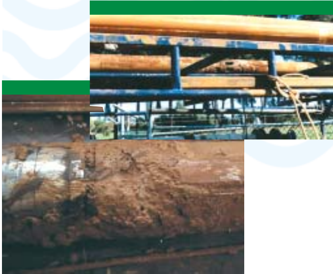
Pump fouling caused by iron bacteria
