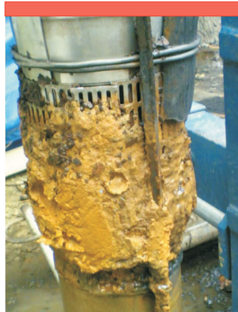
Example of clogged submersible pump
