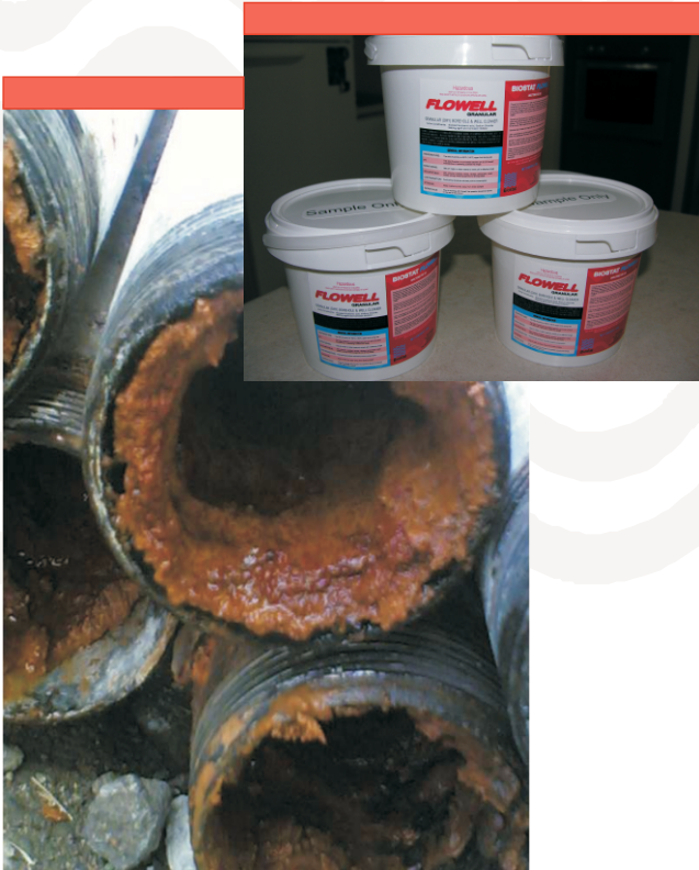
Example of clogged pump discharge pipe
