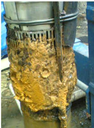
IRB Clogged pump
