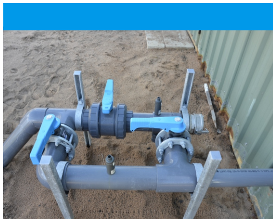
PolyVac Scourer Launch & Retrieval Point
