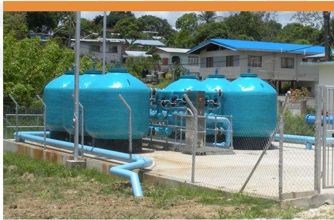
The TIRM DMI65 plants are equipped with high quality valves for flow and backwash control
